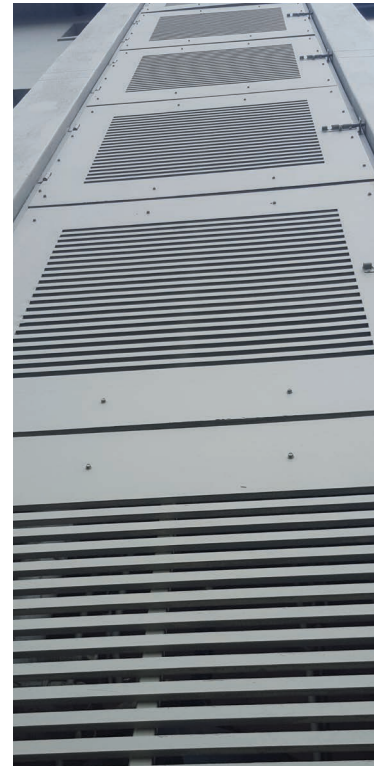
Duct covers on ventilation and services shaft.
